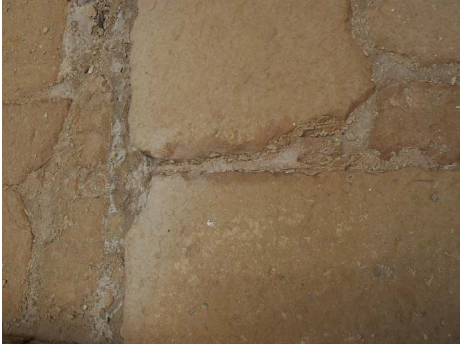
Photo 4 Light, fine crystallized gypsum at species between blocks used as material cementing blocks of Abu Rowash Pyramid
