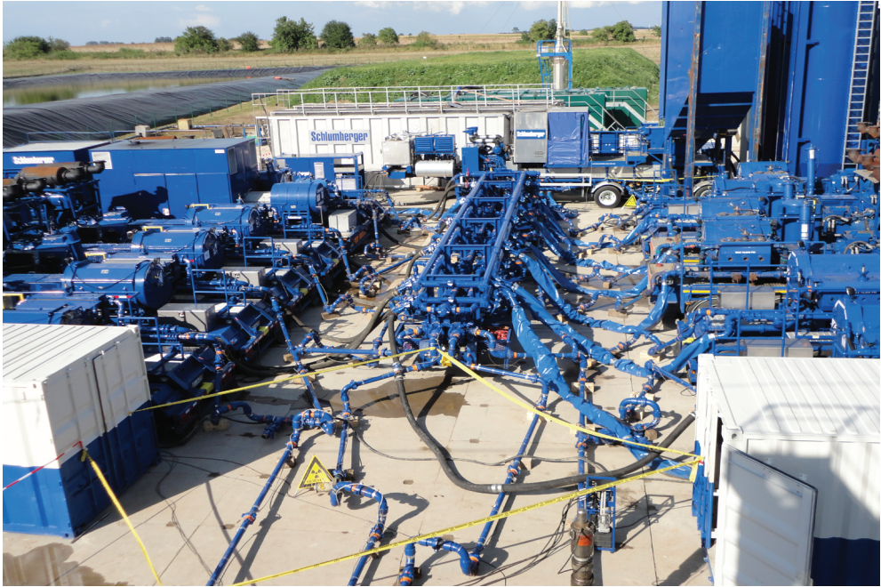
Fig. 5. Interconnected pumping units [4]
