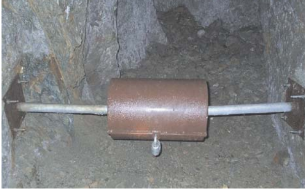
Fig. 2. The TM-71 crack gauge mounted in Janowice Wielkie (phot. S. Cacoń)
