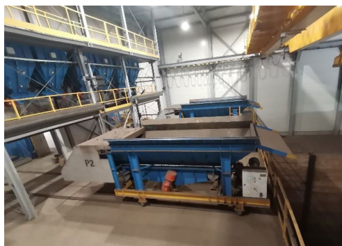
Fig. 1. Automated charge material weighing and dosing system
